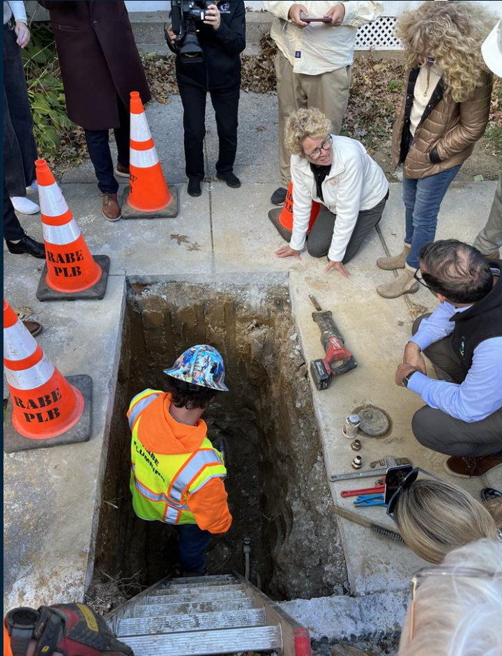
EPA Regional Administrator, Adam Ortiz, joined Chrissy in West Chester to demonstrate lead pipe removal and replacement. This work was funded by IJA.
