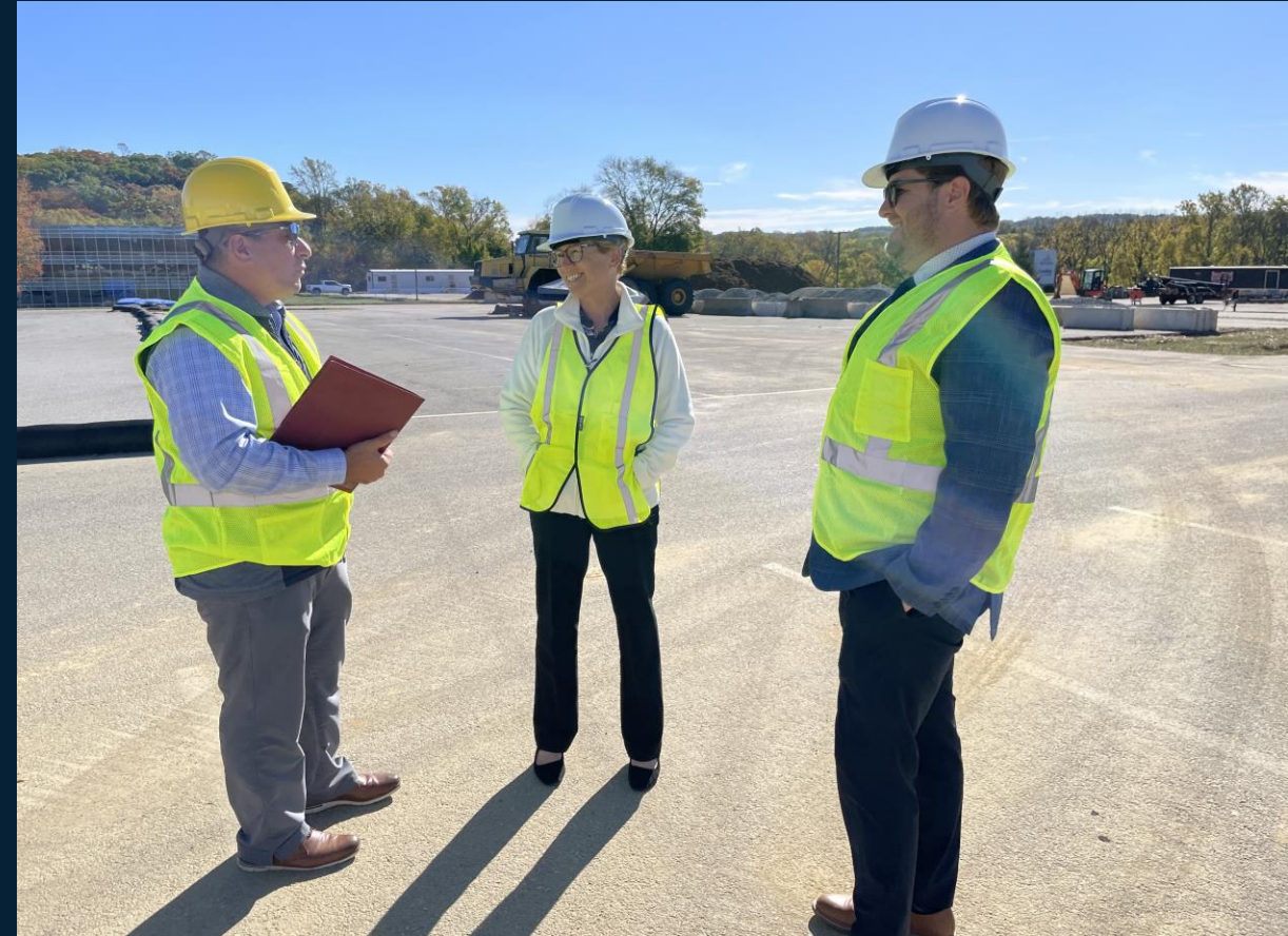
In October 2024, Houlahan visited Chester County Intermediate Unit (CCIU) and the construction site of their new Child & Career Development Center, Great Valley Campus in Malvern. This campus is an extension of their Coatesville Campus and is set to open in September 2026.
